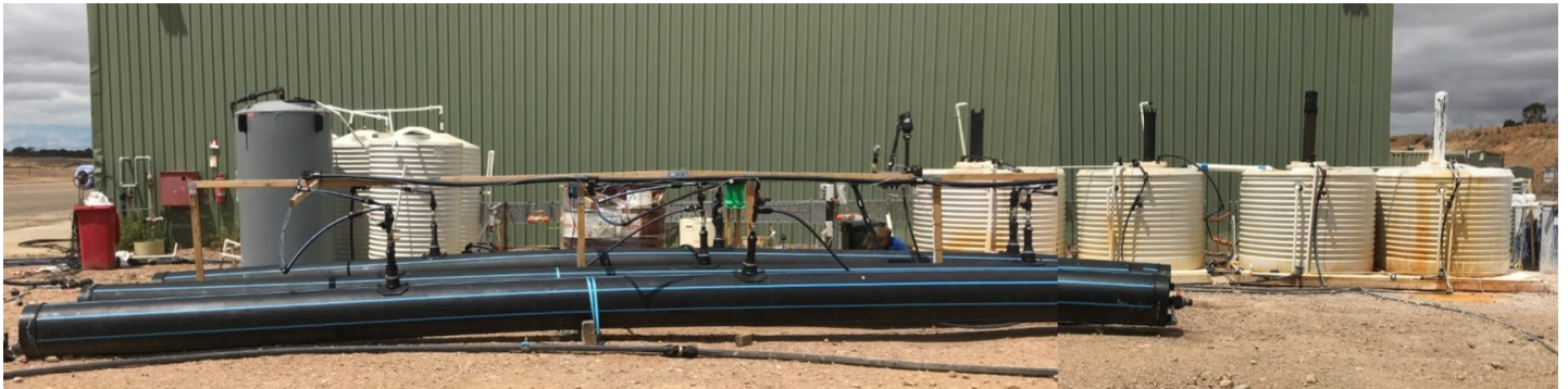
Figure 2. BIO AQUA treatment plant in operation
