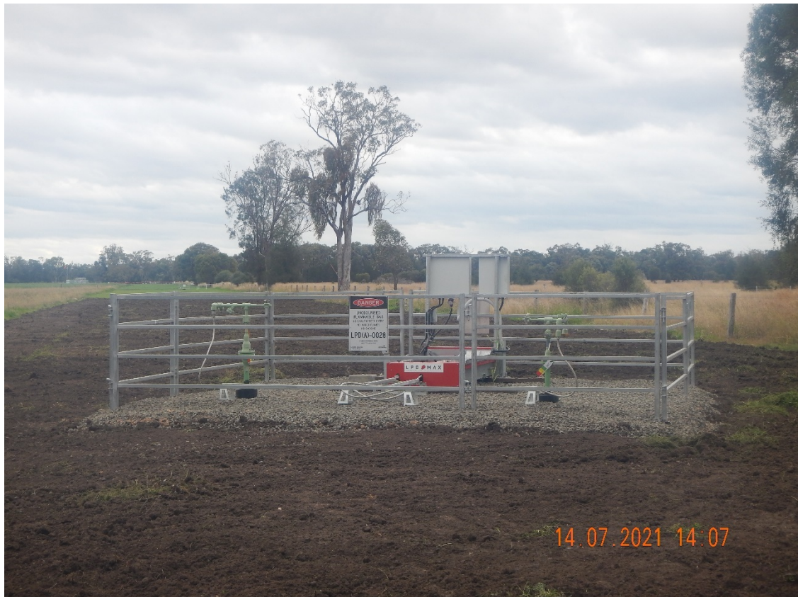
Plate 3-2 - Image a Low Point Drain
