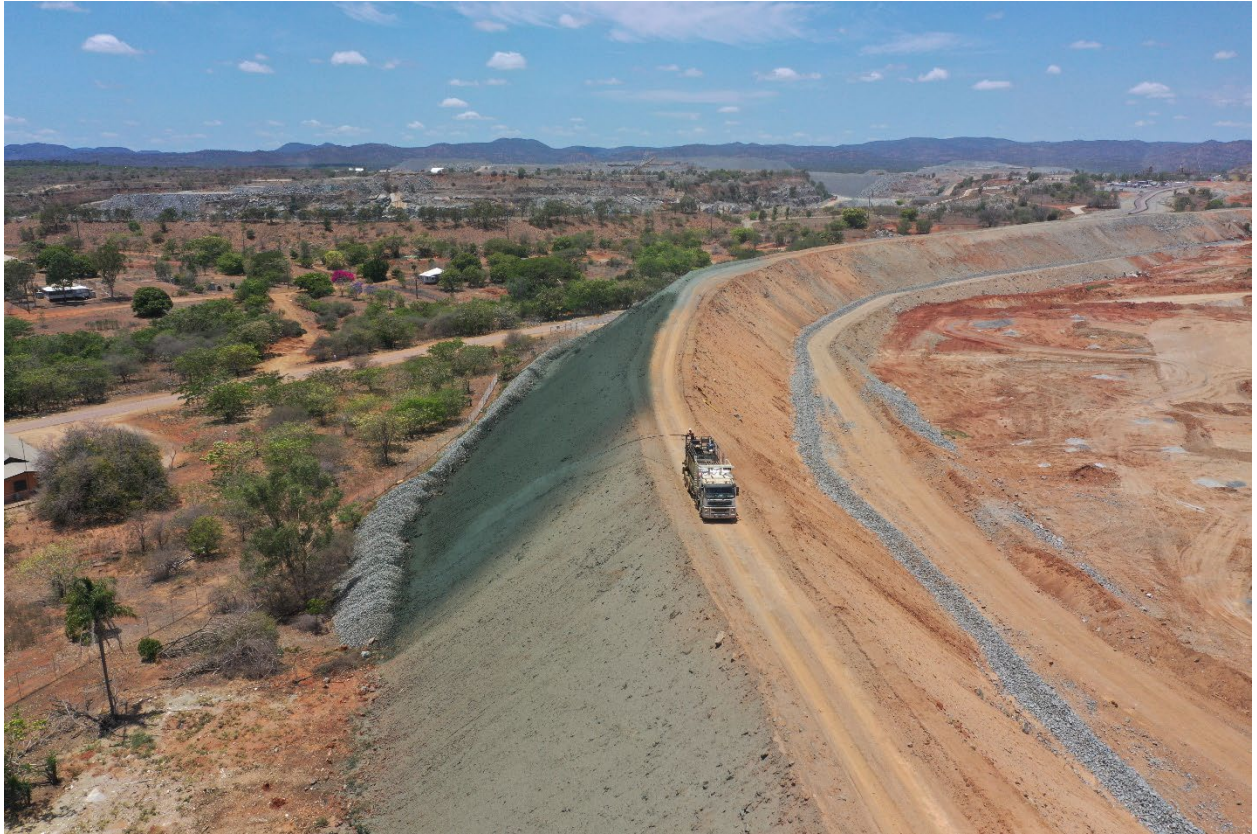
Figure 4. Hydromulching outer batter (community side) of acoustic bund to improve visual amenity.
