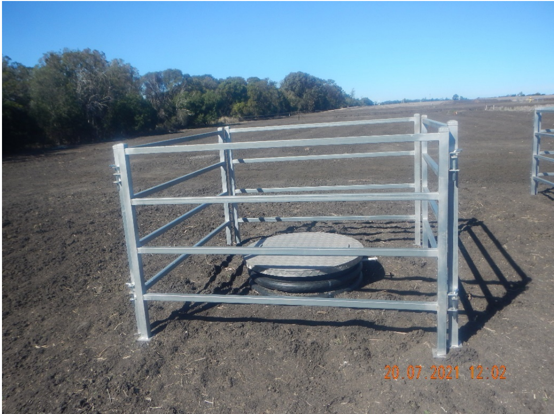
Plate 3-5 – Image of a valve post construction once the ROW has been backfilled
